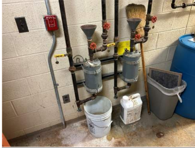
Photo 10: Chemical Bypass Feeders for Heating & Cooling Systems
