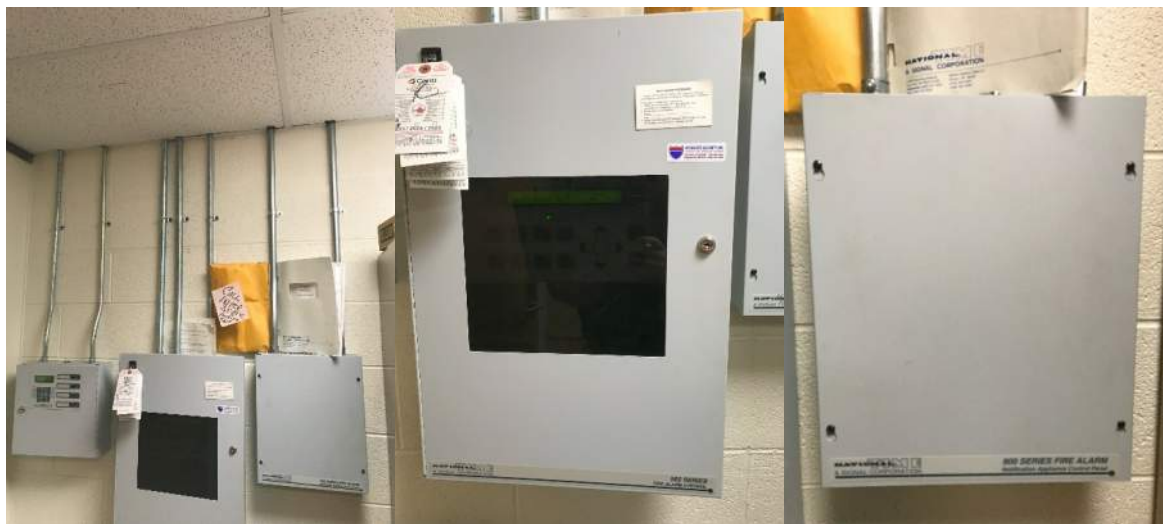
Photo 32: Existing Fire Alarm Panel
