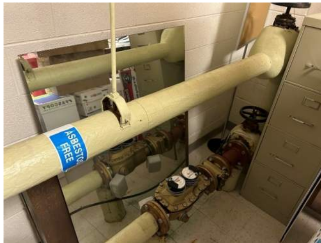
Photo 1: Domestic Water Service
