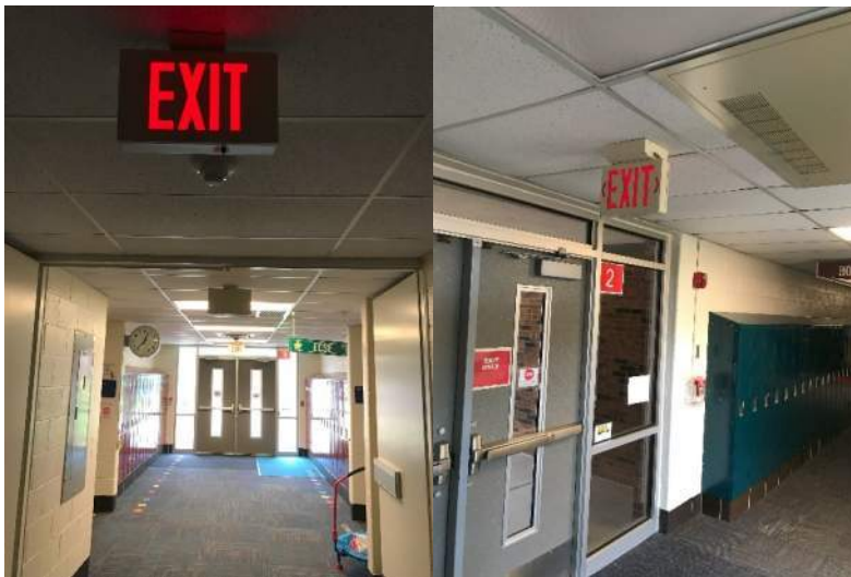
Photo 31: Typical Corridor EBU/Exit Sign
