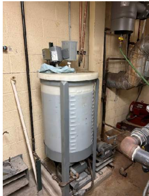
Photo 9: Second Glycol Feed Unit
