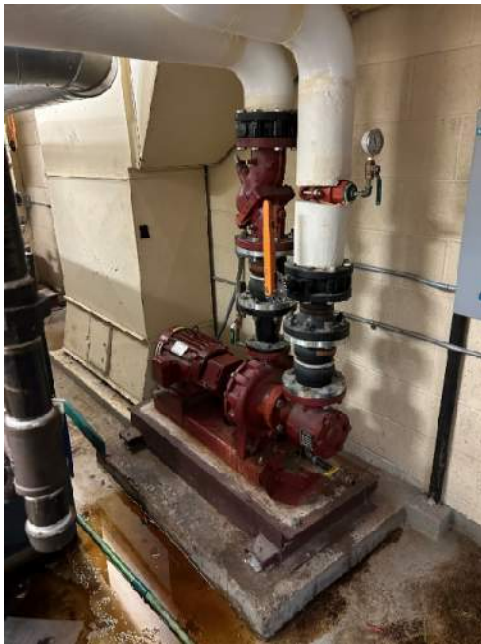
Photo 13: Hot Water Heating Pump
