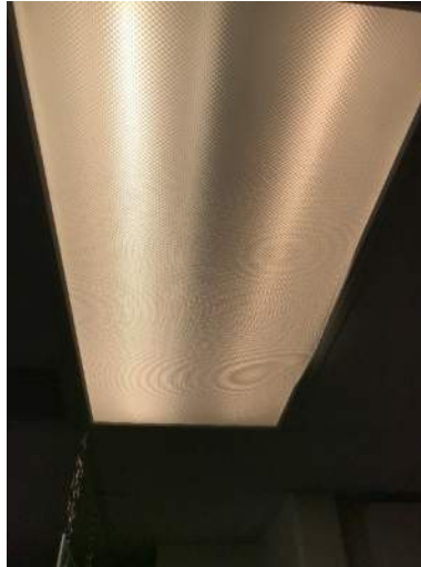
Photo 33: Typical Corridor and Classroom 2x4 Troffer Light
