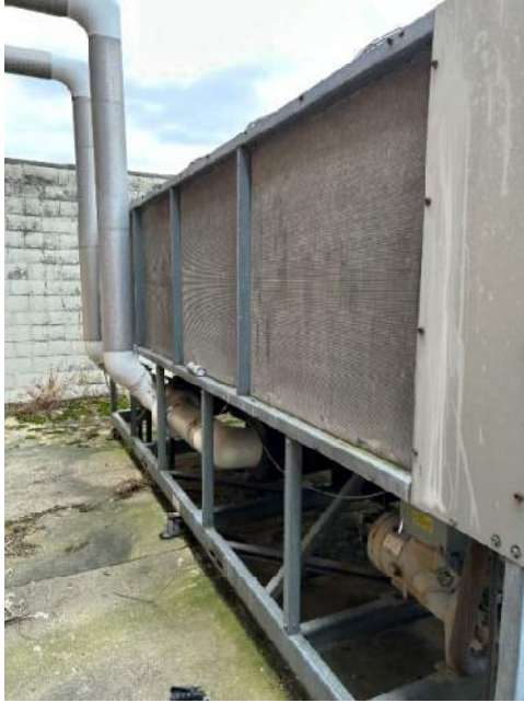
Photo 6: Air Cooled Chiller
