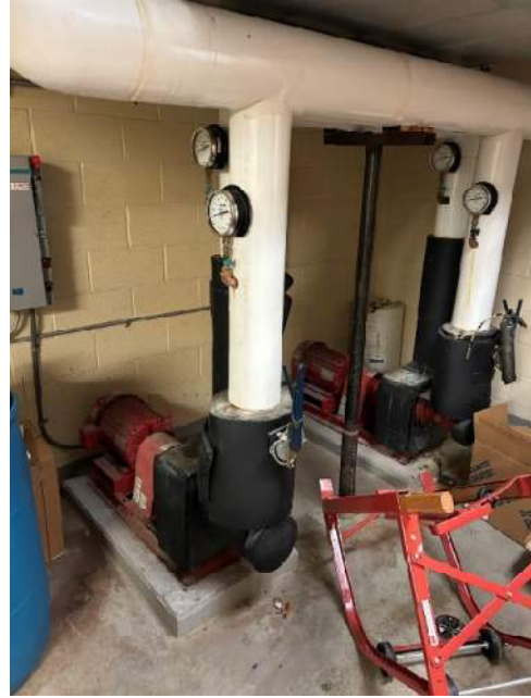
Photo 7: Chilled Water Pumps
