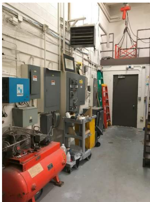
Photo 27: Main Community Center Electrical Room
