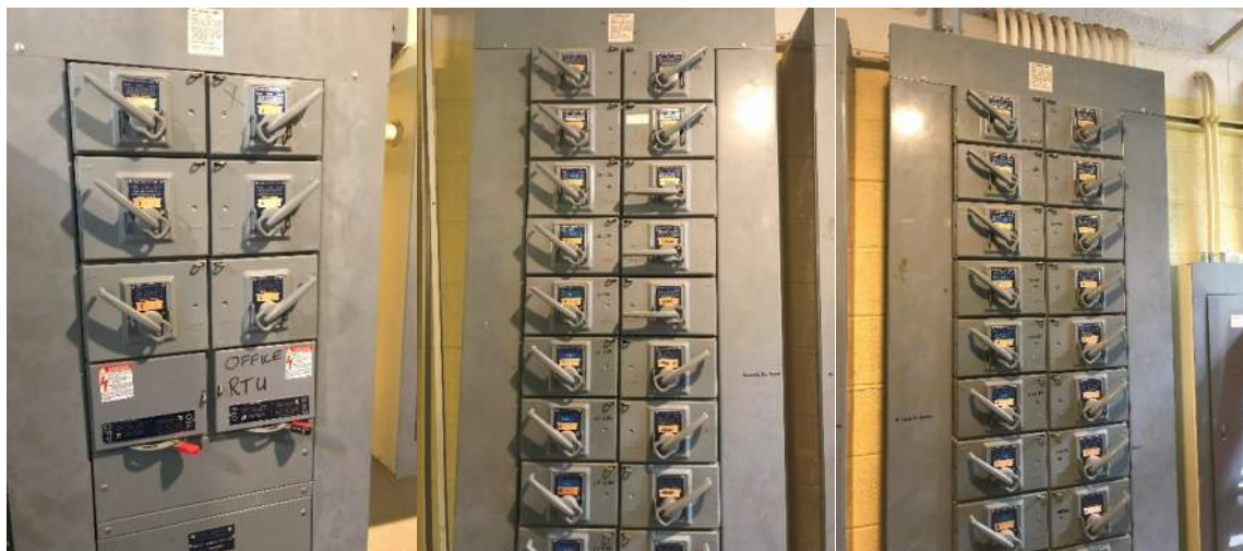
Photo 17: Library and Community Center Electrical Room (DP-2, DP-4, DP-3 respectively)
