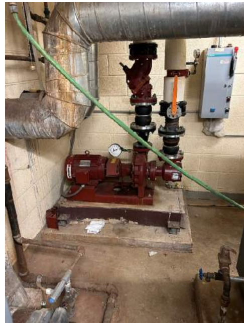
Photo 14: Hot Water Heating Pump
