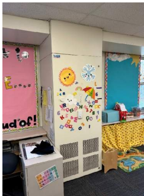
Photo 4: Vertical Unit Ventilator
