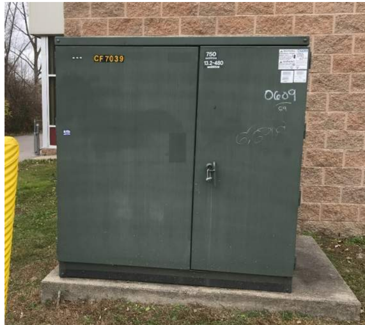
Photo 15: Pad Mounted 750 kVA Utility Transformer
