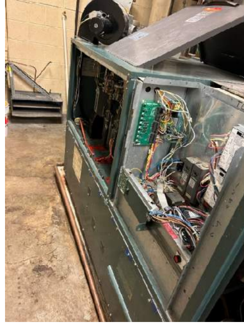
Photo 12: Hot Water Heating Boiler
