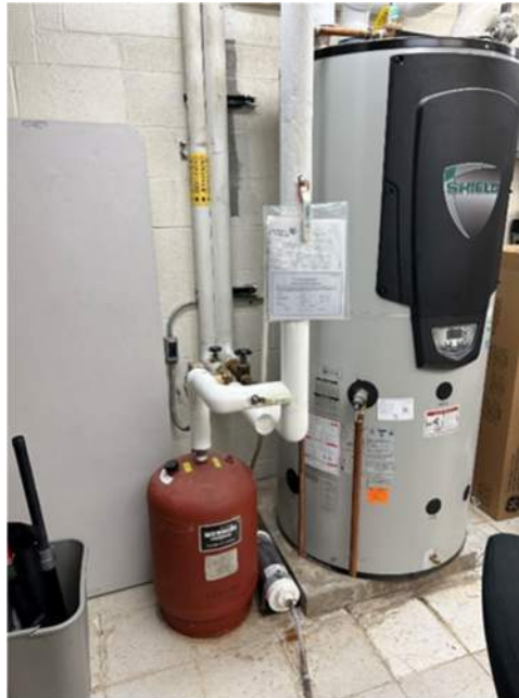
Photo 2: Domestic Hot Water Heater
