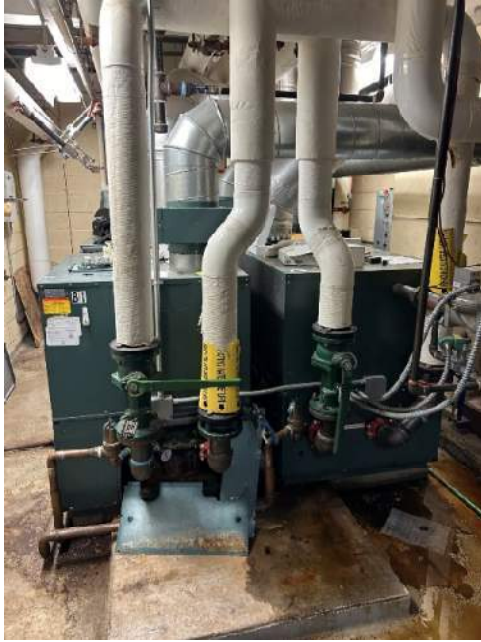
Photo 11: Hot Water Heating Boilers
