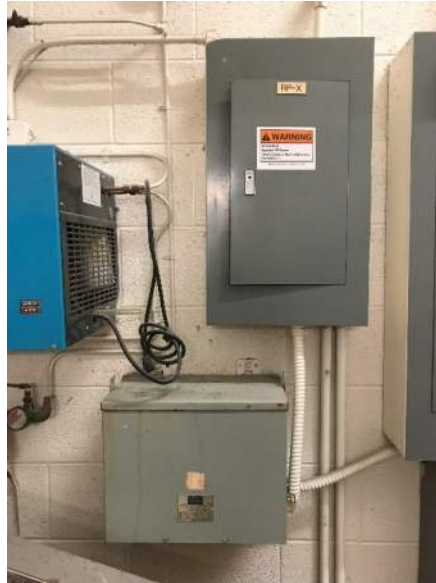
Photo 30: Panel RP-X and Transformer T-X
