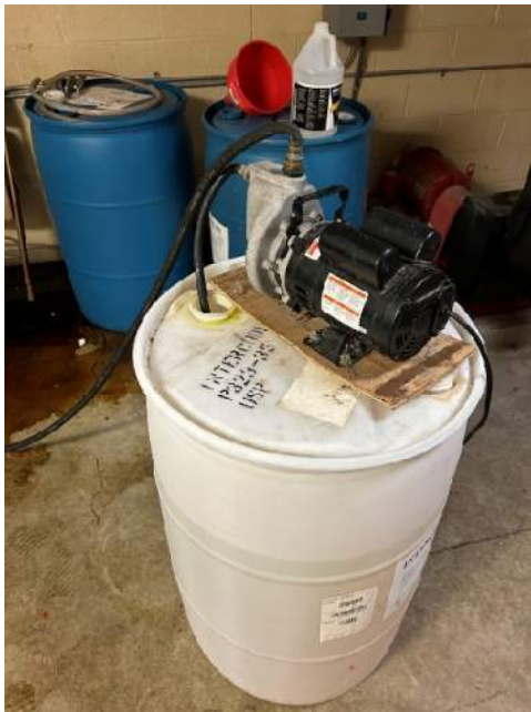
Photo 8: Glycol Feed Unit
